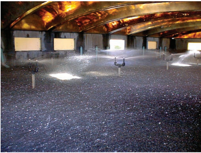
Intermittent sand filter (Secondary Treatment).
