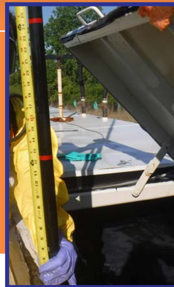
Liquid waste measurement collected during ISTT operation. See Page 1 for more information.
