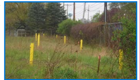
Cluster of piezometers at the Velsicol site. A piezometer is a device used to measure the pressure of groundwater at a specific point.
