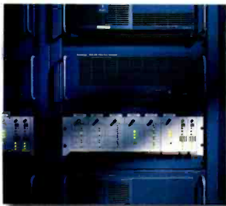
Alamar automation systems are designed to interface with a wide range of video servers including this one at TCI.
