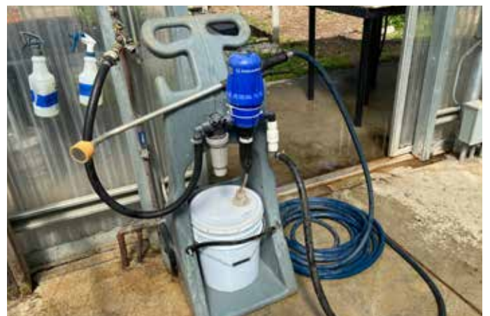
FIGURE 26. Fertilizer injector on mobile dolly with cam-lock fittings so it can be easily connected/disconnected and moved from greenhouse to field and back. Photo: Christof Bernau
