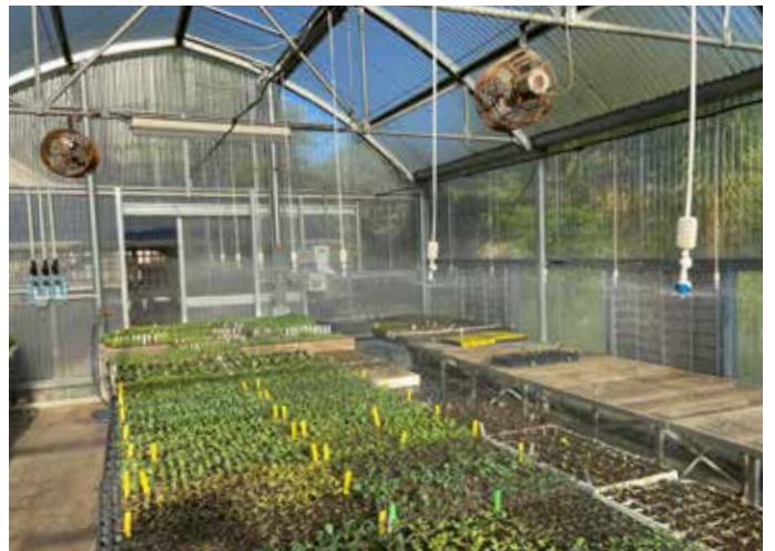
FIGURE 23. Typical 3/4" solenoid valves with screen filters to prevent debris from clogging sprinkler nozzles. Three bench, three valve layout, controller in right rear of photo, valves for each station in left rear of photo and sprinkler nozzles arrayed evenly over each bench to provide uniform water delivery. Photos: Christof Bernau
