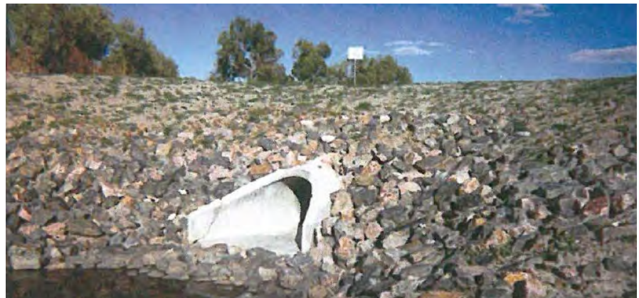
FIGURE 6.11.27 Unprotected Culvert Outlets Cause Downstream Erosion
