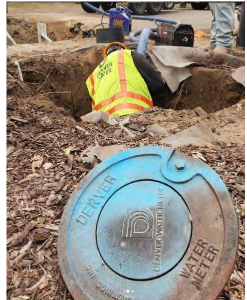
Denver Water’s Lead Reduction Program will replace between 64,000 and 84,000 lead service lines from our water systems.
