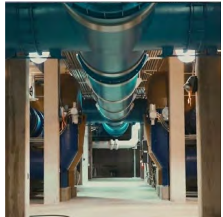
Marston Treatment Plant is one of three drinking water treatment plants that serve 1.5 million people in the Denver-metro area. The plant can treat up to 250 million gallons per day.
