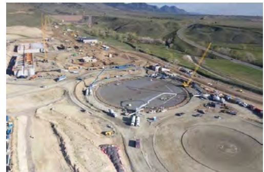
Denver Water’s new, state-of-the-art Northwater Treatment Plant being built between Ralston Reservoir and Highway 93 (seen on the right).
