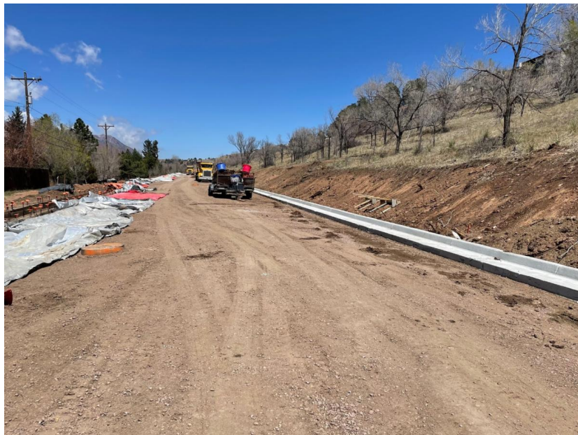
Curb and gutter are now in place along 30th Street between Gateway Road and Fontanero Street
