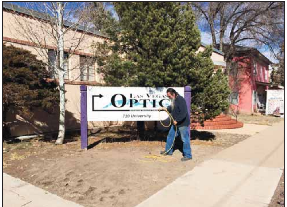
Mike Martinez of Frugal Signs installs the new Optic signboard printed for the Company. His wife and business partner Theresa Martinez was a former inserter for the Optic until 2012 when the press shut down.
