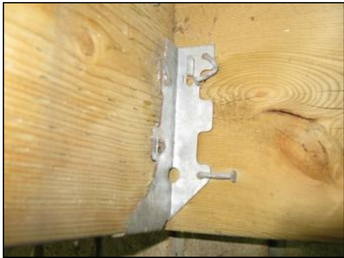
4. Poor end bearing, joist hanger connections
