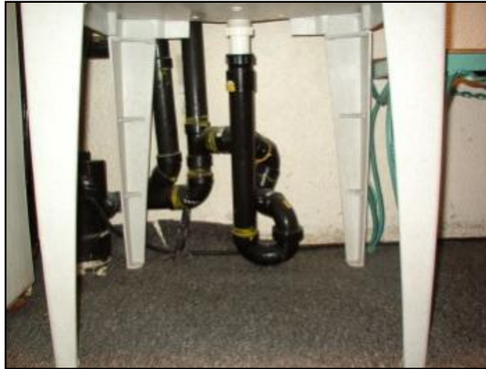
14. Poor trap arrangement
