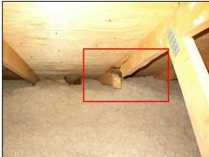
6. Top chord of truss is broken
