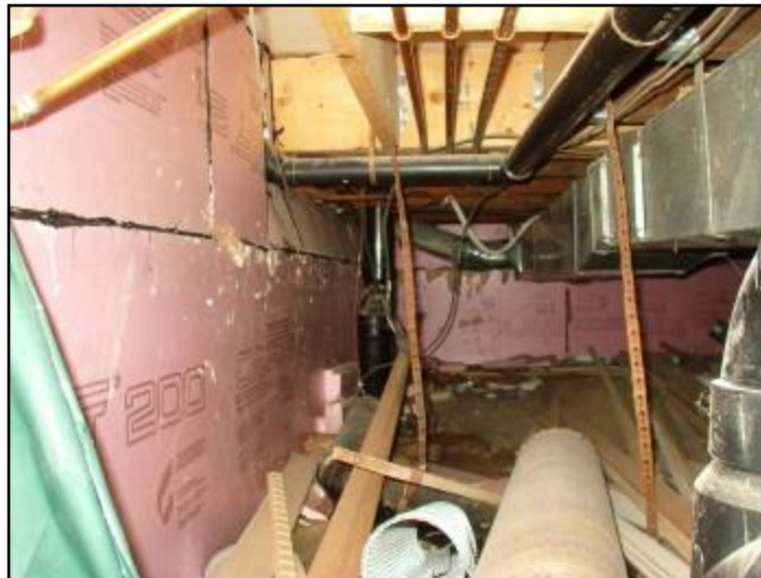
12. Exposed polystyrene insulation is fire hazard
