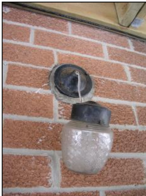
8. Light fixture is not well secured
