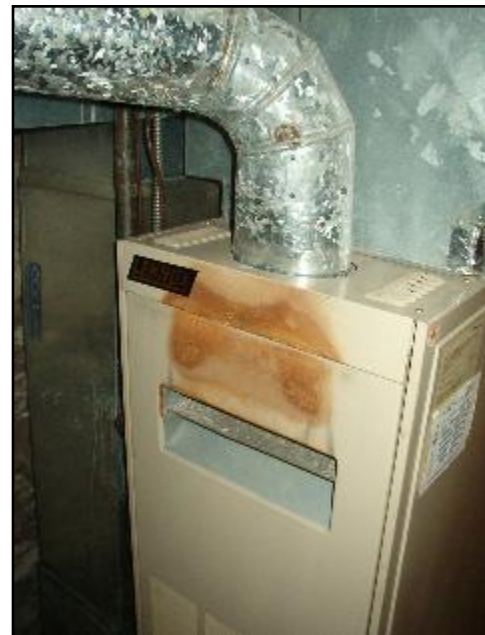
10. Evidence of furnace backdrafting
