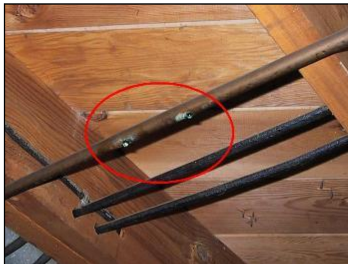
13. Leaking copper supply pipe
