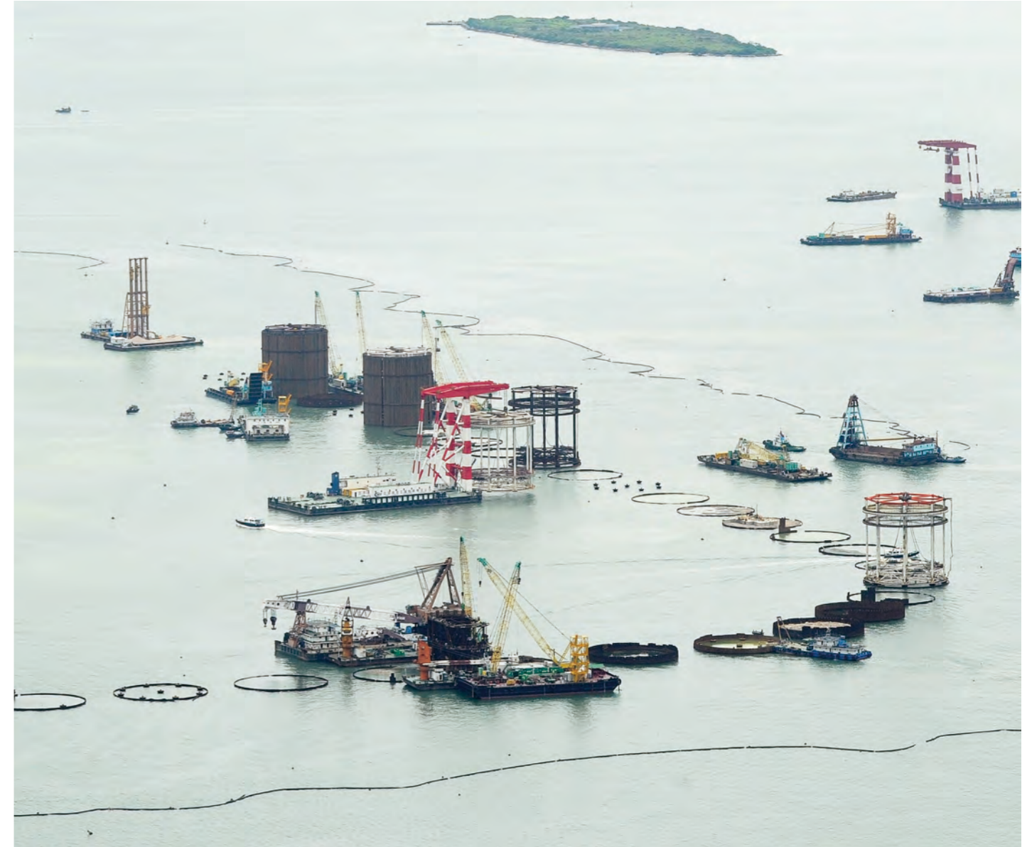
Steel Sheet Pile Cell (Straight web-type sheet pile) Hong Kong Macau Artificial Island / Hong Kong
