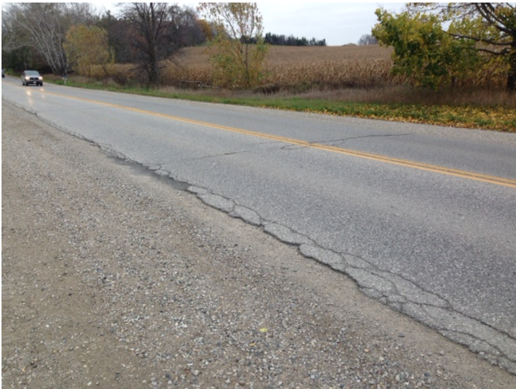
Photograph 8: Conditions along pavement edge, Section 2.
