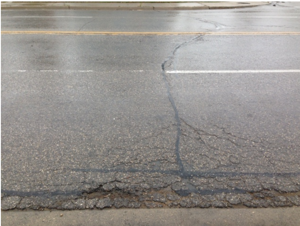
Photograph 10: Conditions along pavement edge and transverse crack, Section 3.
