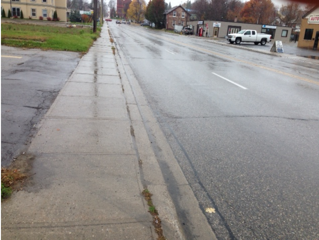
Photograph 11: Section 3, general pavement conditions near Queen Street.
