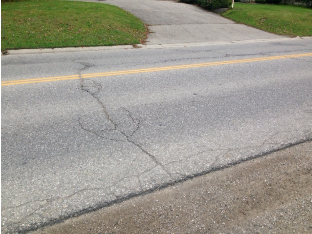
Photograph 7: Section 2, transverse and longitudinal cracking.
