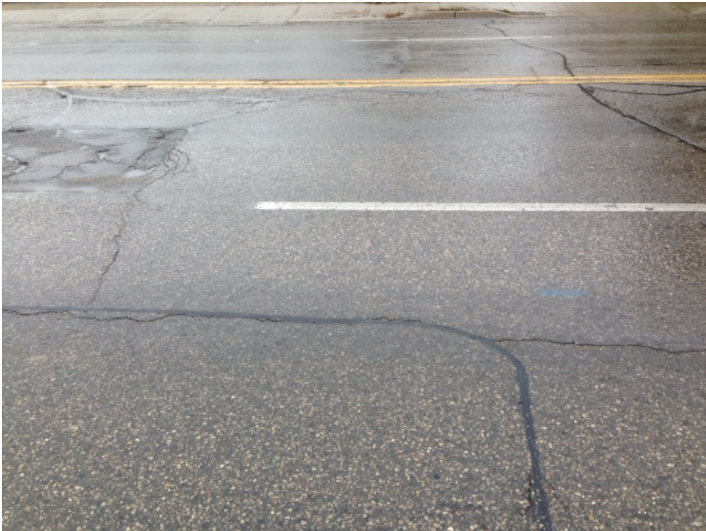
Photograph 12: Severe cracking along Section 3.
