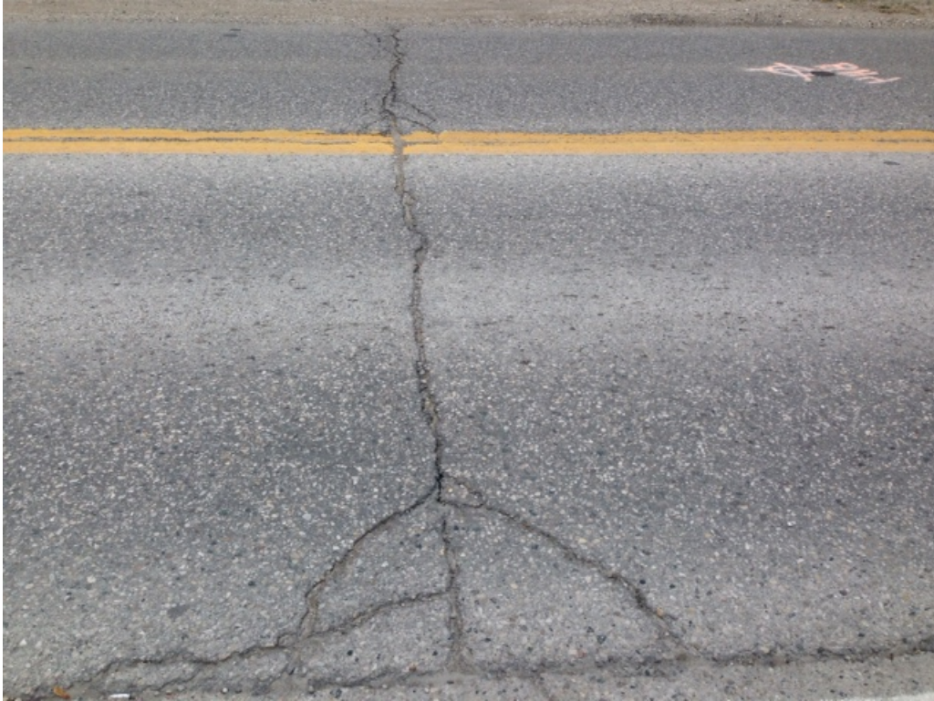
Photograph 5: Section 2 (near BH 4) transverse cracking.
