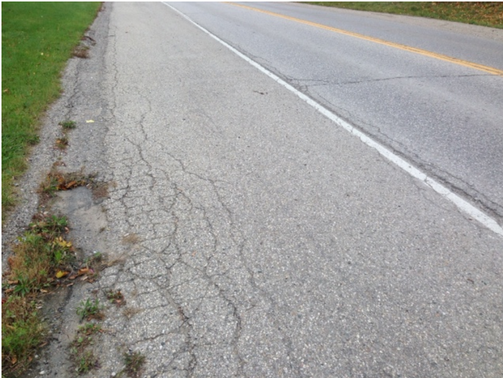
Photograph 6: Alligator cracking along pavement edge, Section 2.
