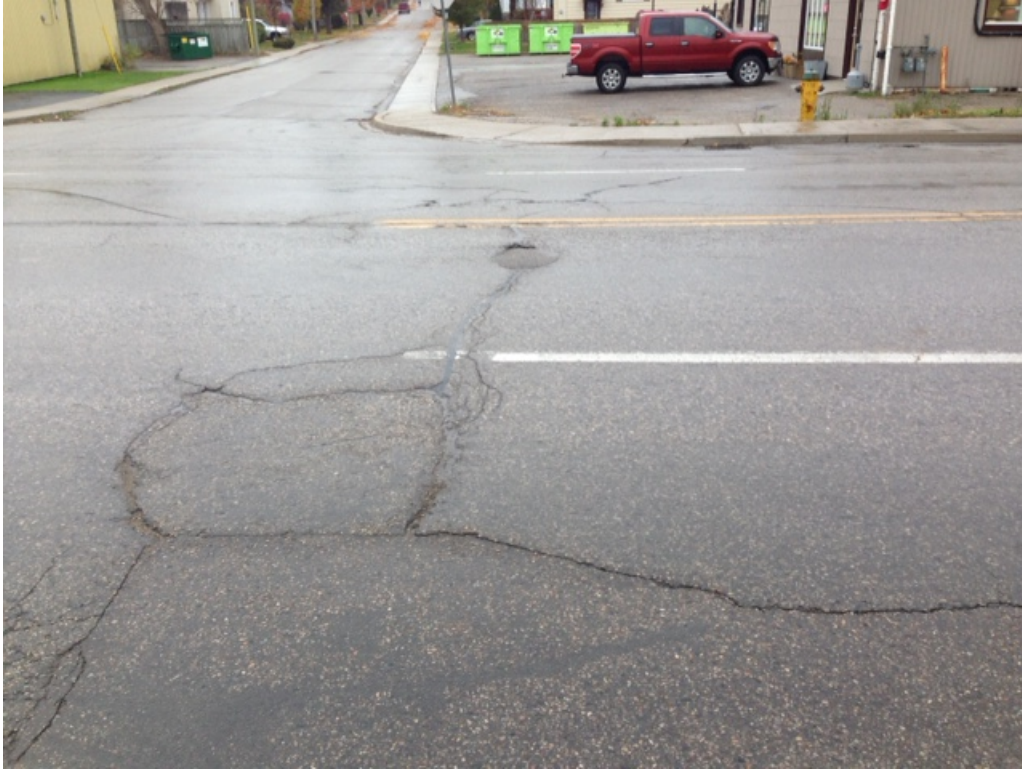
Photograph 9: Section 3, transverse and longitudinal cracking.
