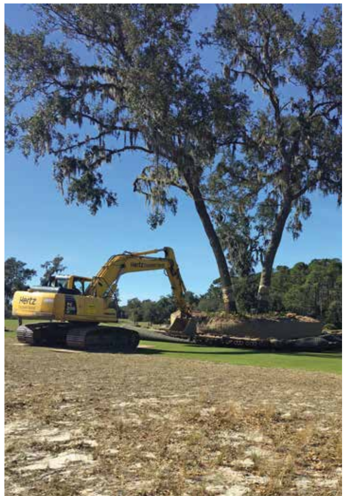
Trees creating shade issues can sometimes be relocated to another site on the golf course. Photo credit: Jon Hatten.
