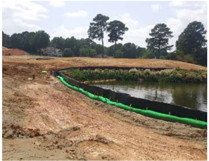
Silt fencing during construction projects is a critical element of BMPs to prevent erosion and sedimentation. Photo credit: Brandon Hayes.
