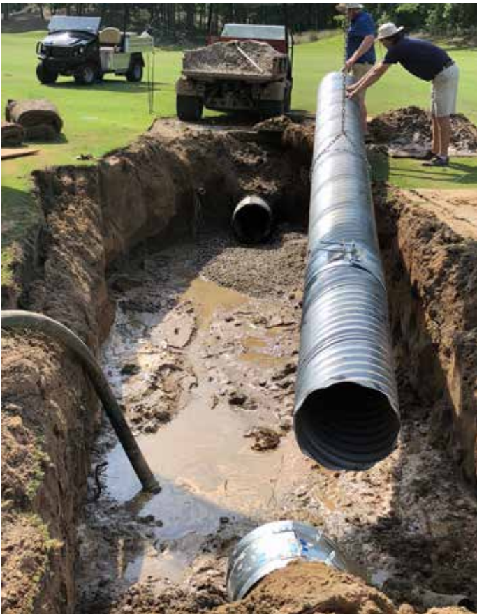
Drainage systems should be routinely inspected to ensure proper function. Photo credit: Ronald McWhorter.
