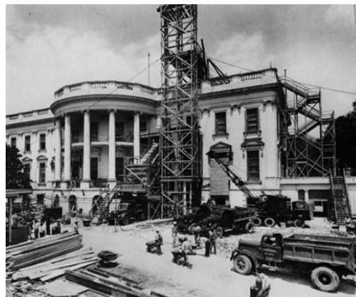
In 1952, renovation and reconstruction of the White House was completed. Two new levels were added below ground and, at Truman's request, a balcony was added to the south portico.
