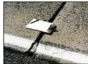
Faulting (JPCP Only)
