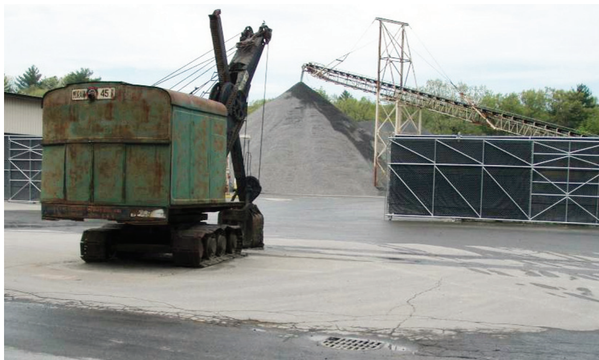
Storm drain adjacent to access road to plant; drain is not protected and not being serviced.
