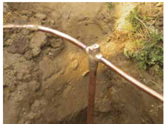
GT Cadweld connection
