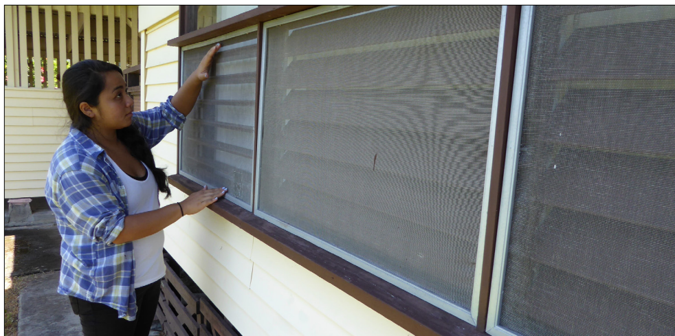
Mosquitoes will find holes and cracks in a screen and sense our body's carbon dioxide, so keeping doors closed and screens in good repair can prevent indoor bites.
