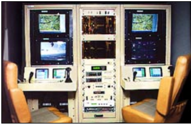
Figure 11. Predator ground control station layout.
