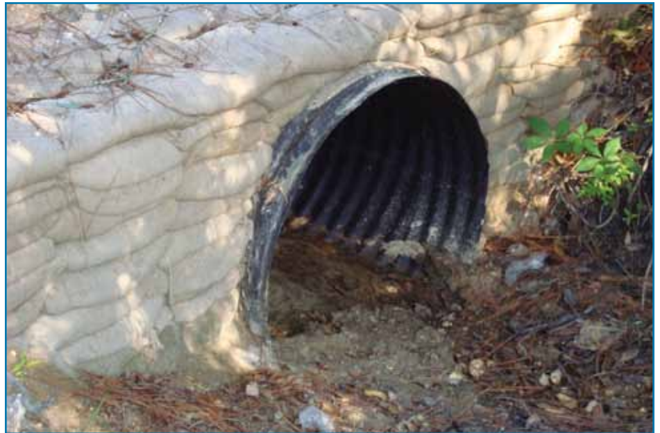
Figure 3.2-4. Culvert with sandbagged headwall is being used in a sandy soil drainage ditch. This method should not be used for permanent use in water courses.
