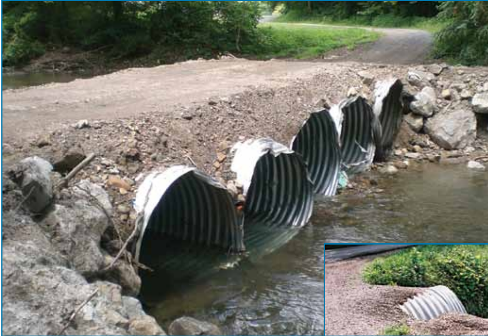
Figure 3.2-2. This multiple culvert crossing is vulnerable to debris blockage and washout. To install multiple or a “gang” of culverts properly, each culvert must be spaced adequately to allow for proper soil compaction between the culverts. This fill must be well armored at each end to prevent the washing out between the culverts.
