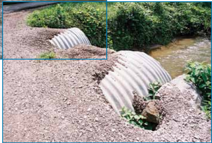
Figure 3.2-3. (right) Insufficient cover for culverts will result in washout and erosion as well as structural failure and collapse of culverts.
