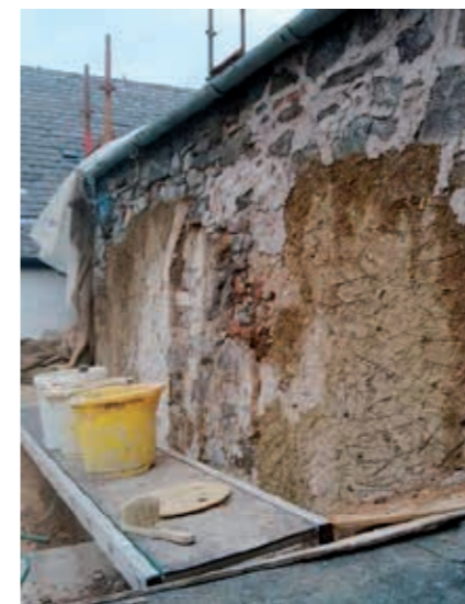
Gray House, a mudwall building in Errol, was refurbished and restored as part of the Tay Landscape Partnership project.
