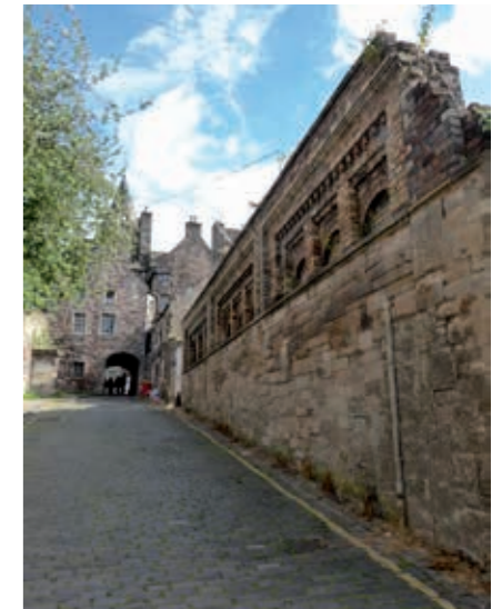
A rare survivor of Canongate's industrial past: a boundary wall at threat of being demolished in order to create an eight-storey student residence behind the iconic Tolbooth. © Jilly MacLeod
