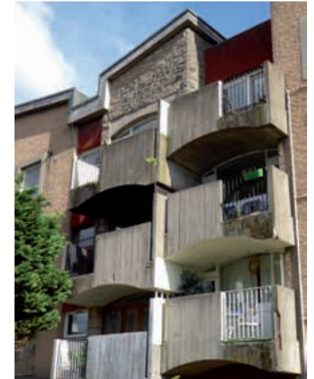
The Basil Spence flats, Cannongate, Edinburgh have had several applications for replacement windows: some uPVC, others losing original opening methods and design. © Jilly MacLeod
