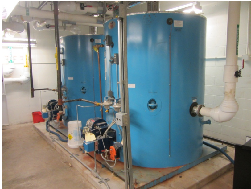
4: Two 600 gal domestic hot water boilers with 80% efficient burners
