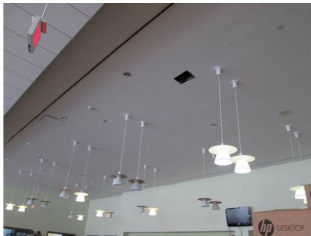
7: Decorative atrium lighting
