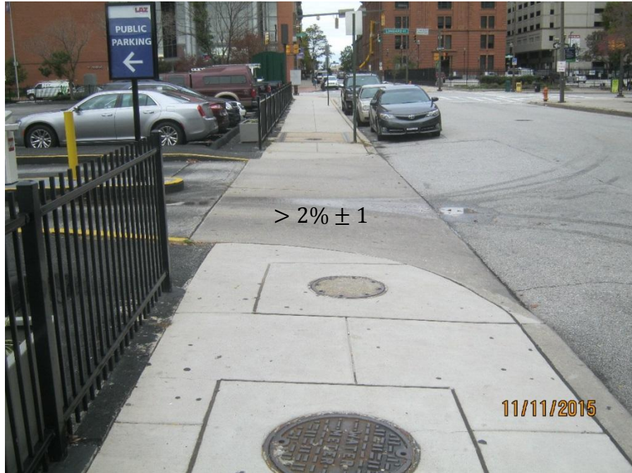
Non-compliant Driveway: The cross slope at the entrance of this surface parking lot has a slope that exceeds the maximum 2%.
