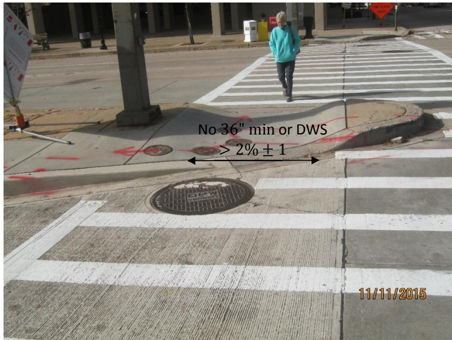
Non-compliant Median Treatment: A pedestrian refuge island, also known as median cut-throughs, shall also be equipped with detectable warning surfaces at its edges.
