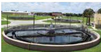
Palm Beach County Aeration Facility
