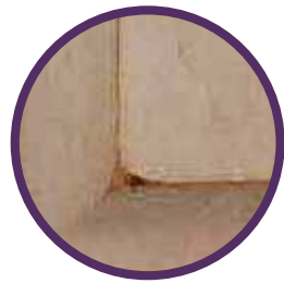
Over-sanding on areas of unfinished door and drawer fronts 1
