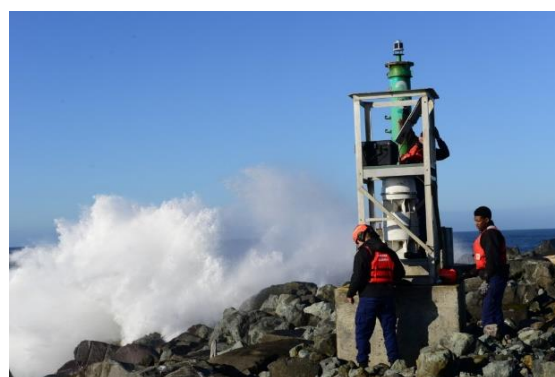
Crew members from Aids to Navigation Team Astoria service a foghorn at the end of the Tillamook River North Jetty near Garibaldi, OR.
