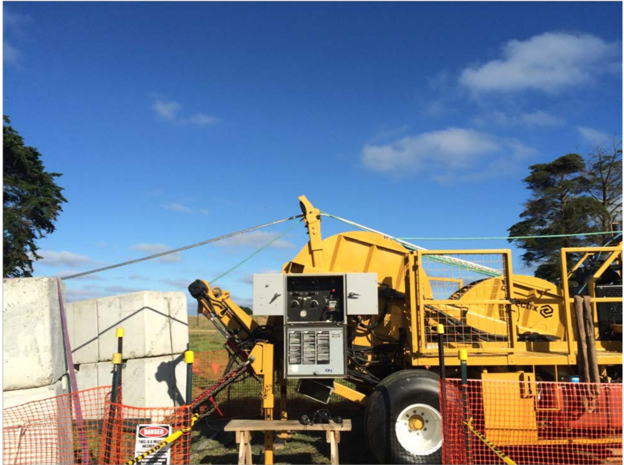
Figure 1: Example of a situation where bending is excessive even for ACSR. In this case, the payout reel is located downslope from the bull wheel, and the conductor bending angle is 35^{\circ} around a four (4) inch roller. Photo courtesy of Trans Power New Zealand.
