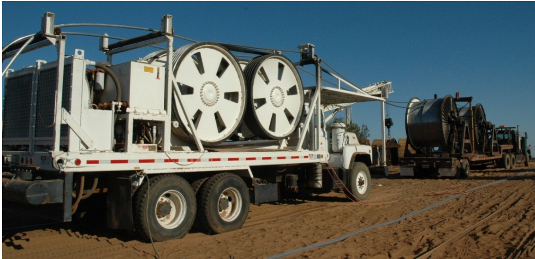
Figure 11: Dual drum bullwheel, courtesy of ONCOR Power Delivery.
