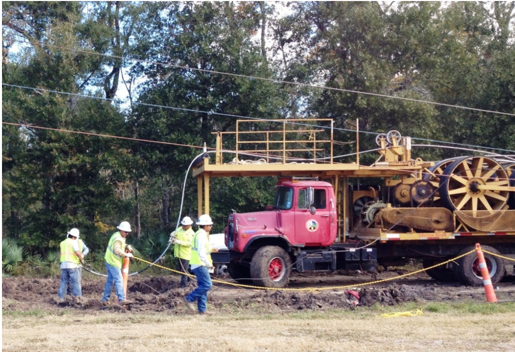
Figure 4: It is OK to drape slack conductor across a small roller. This would not be acceptable if the conductor was under tension or if the crew was pulling the tail to install a fitting.
