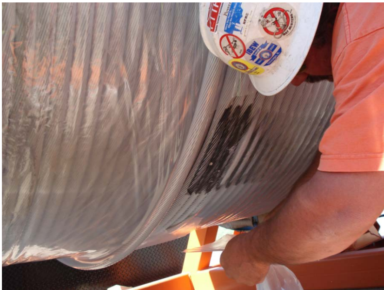
Figure 25: Water stain on conductor.
