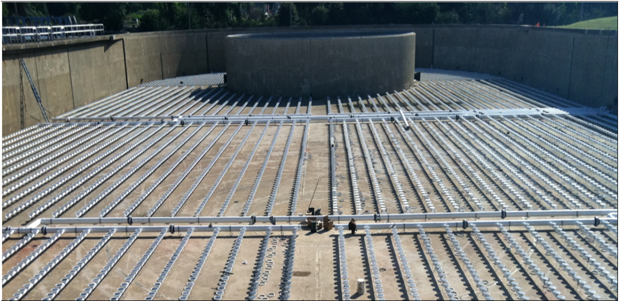
Figure 2: Construction of the fixed disc diffuser array. (Tony Fitts, Jackson Energy Authority)
