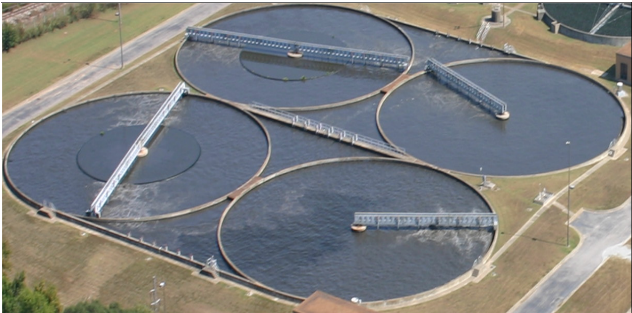
Figure 1: The Schreiber Counter Current Aeration System featuring anoxic center rings, tandem bridges (left), and single bridges (right). (Cassandra Fuller, Jackson Energy Authority)
