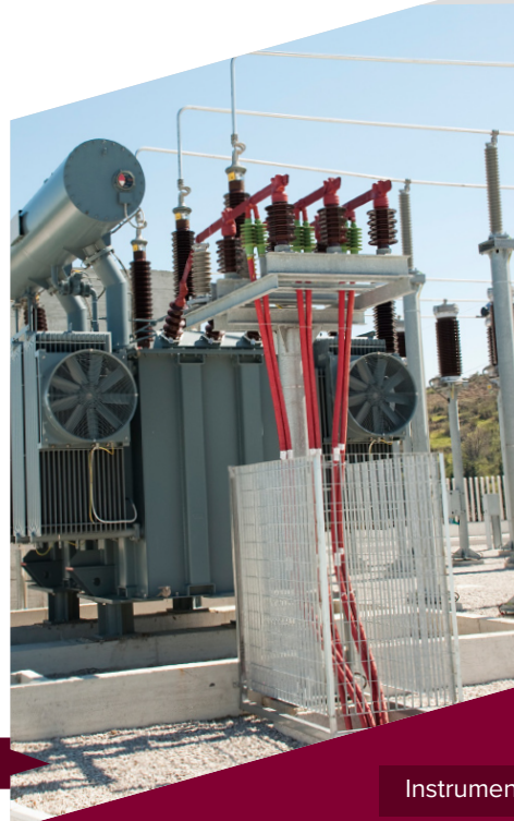
High Voltage Services
