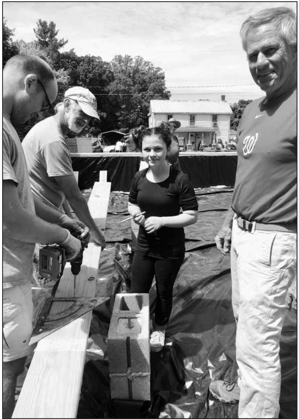
Some people take the opportunity during a weekend to give back to their community. The Farmville Area Habitat for Humanity volunteer group meet on Camden Street in Dillwyn to work on the foundation of a new house in the process of being built. Volunteers Don Williams, Danielle, Ryan Mast (of Americorps) and Chris Yates are shown working on part of the foundation of the new home being built. If you're interested in volunteering for this very worthy project contact the area office at 434-394-3001.
