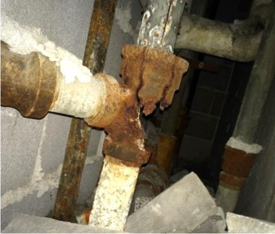
Completely rotted pipe
