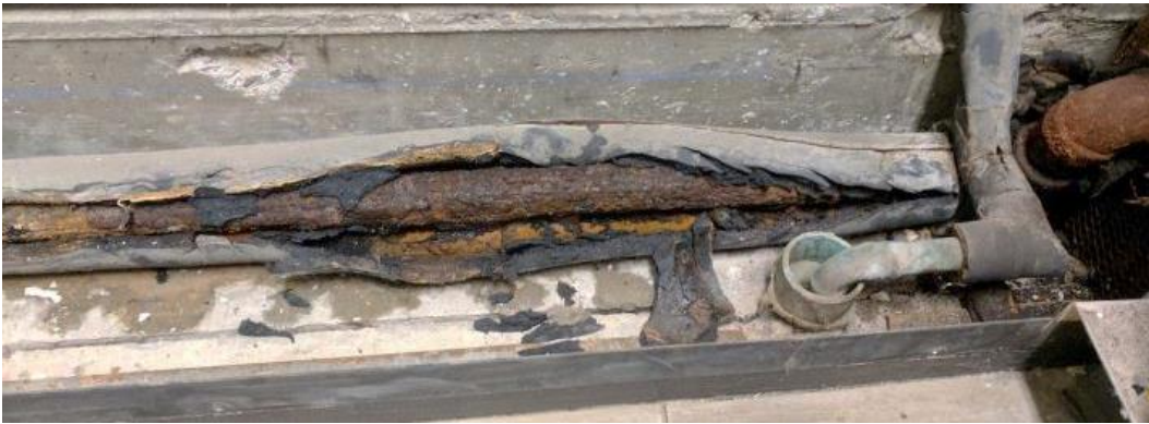
Pipe casing damage
