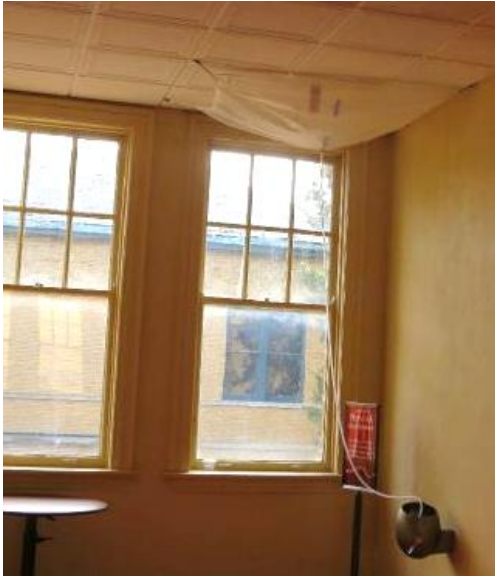
Ceiling leak (with improvised drainage system)
