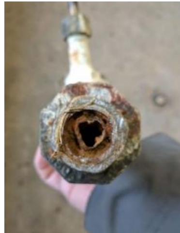
Internal pipe damage
