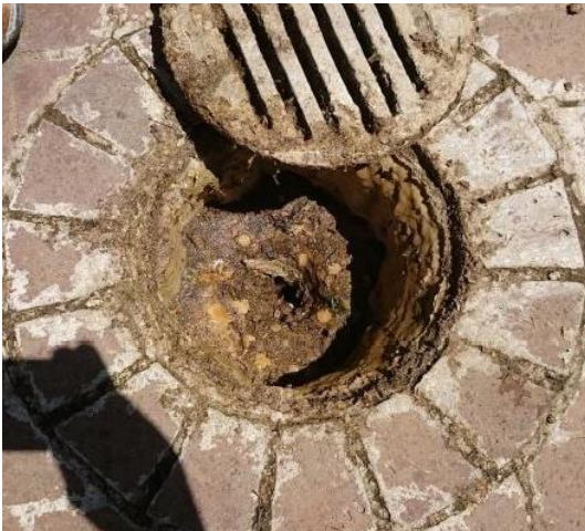
Internal drain damage
