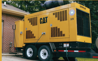
Permanent or portable generators
