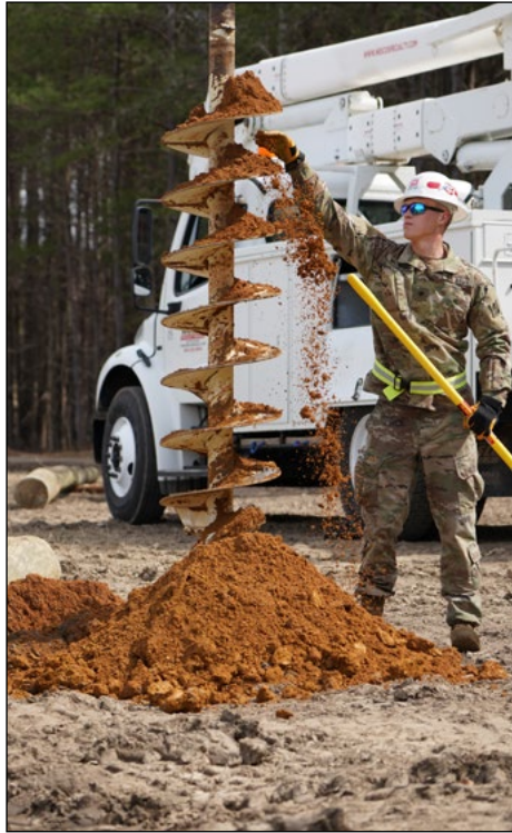
(Photos by David Gray) Power distribution specialists supervise drill digging for the installment of a power utility pole during a recent field training exercise at Fort A.P. Hill, Virginia.
