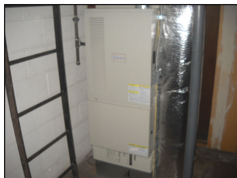
Newer furnace unit.
