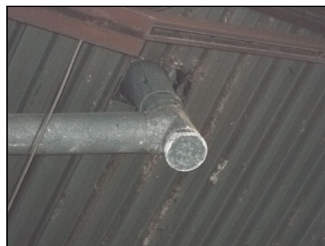
Evidence of roof leakage at chimney protrusion.
