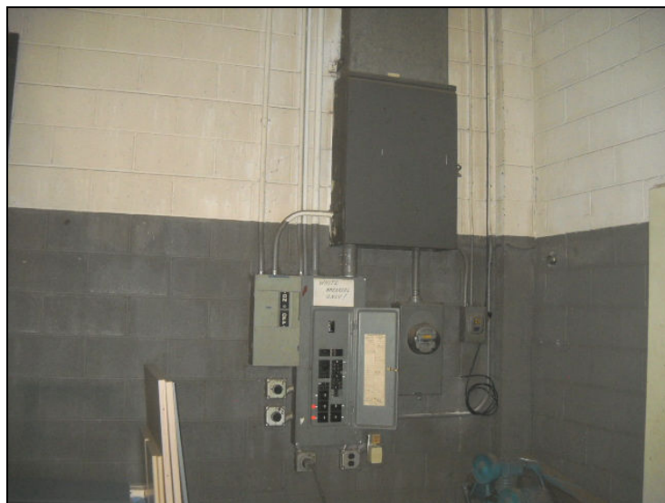
Electrical service for the north suite.
