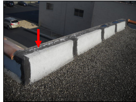
Missing coping on parapet wall.
