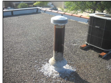
Surface corrosion on chimneys.
