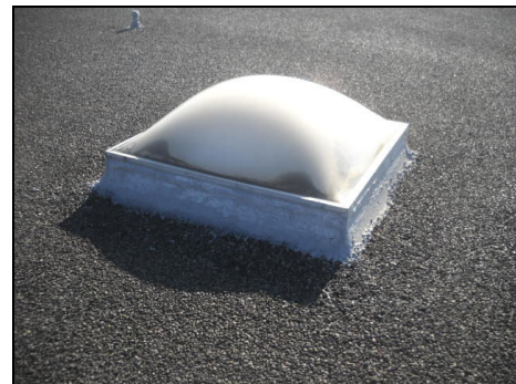
Skylight flashing needs caulking.
