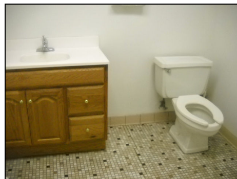
Representative view of bathroom fixtures.
