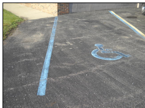
Present, yet insufficient ADA parking.
