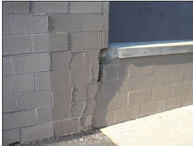
Block and cap damage at retaining wall for truck well.
