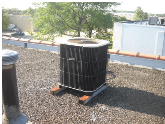
Older condenser unit serving west side.
