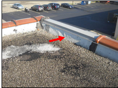
Loose material at parapet wall.
