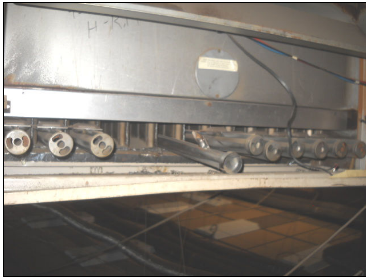
Unitary heating system partially dismantled.
