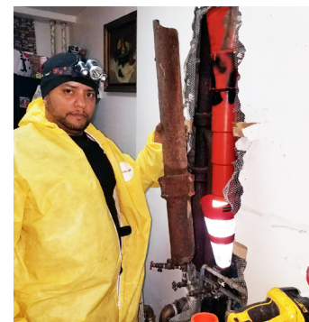
ESD Maintenance Worker Alberto Fellicia recently made an emergency replacement of a rotted pipe to stop a leak until plumbers were able to respond.
