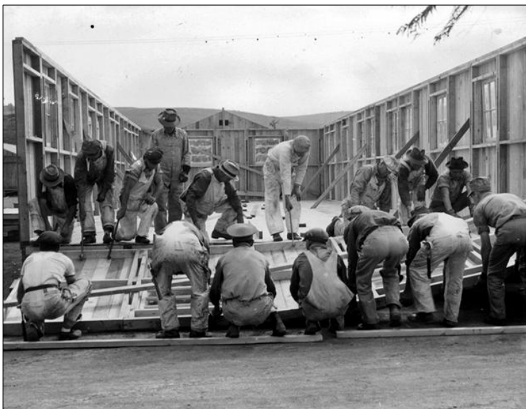
Barracks are being constructed at the Los Angeles County Fairgrounds at Pomona. WRA photo by Clem Albers, April 8, 1942 Courtesy of the U.S. National Archives and Records Administration
