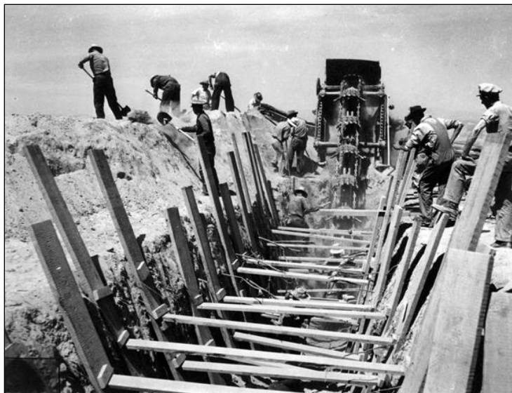
Workers of Japanese ancestry are using a ditch-digging machine to excavate for water pipes and sewer lines at Poston. WRA photo by Clem Albers, April 9, 1942 Courtesy of the U.S. National Archives and Records Administration
