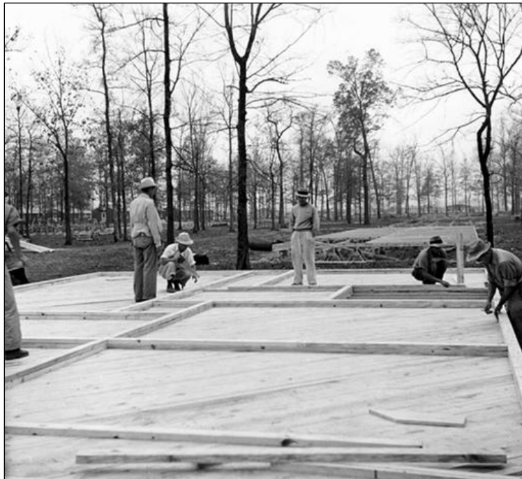
Apartments are being built for the administrative staff at Rohwer in this 1942 photo. The wood frame construction made it fairly easy to remove the buildings after the war, so the land could be returned to cultivation.
