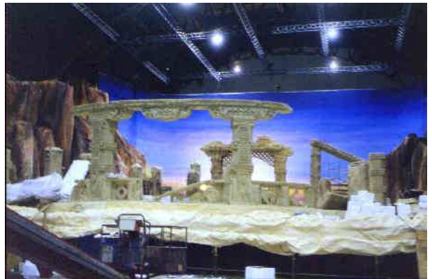
"Phaedos Outlook" was the last large scale set to be constructed at the showgrounds in what is now, 20 years later, known as Fox Studios Stage No. 7.
