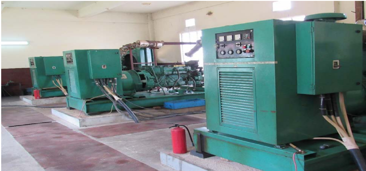
Power generators at JFD.
