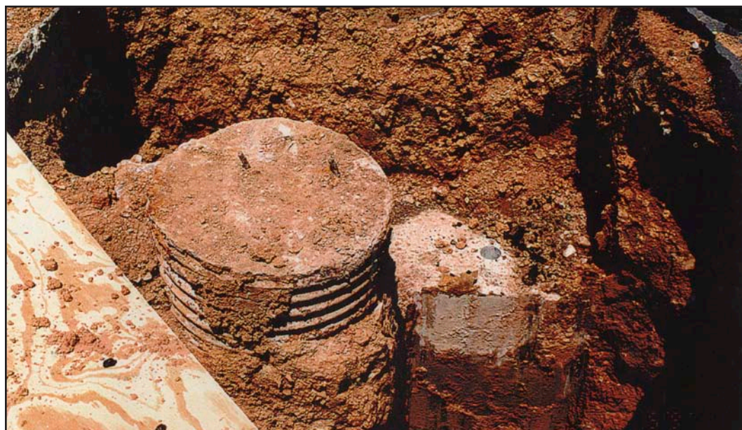
One of the 1,600 Raymond piles beneath the hangar foundations exposed during a 1997 inspection.
